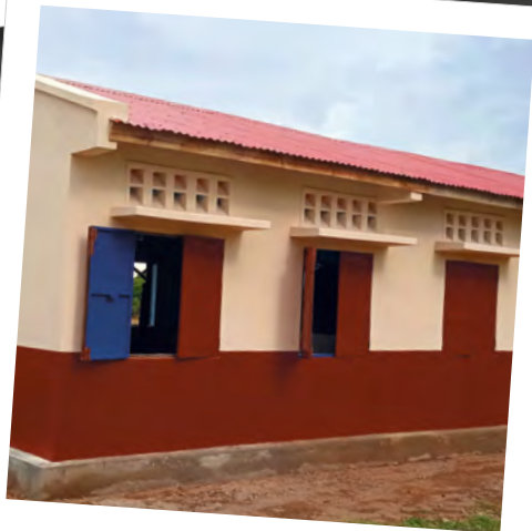
New elementary school construction in Mirafy village, a rural municipality of Ejeda.
