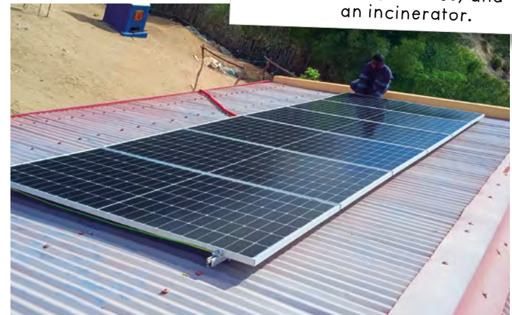
Photovoltaic system installed for Electrical Power in 4 CSBs I: Ampitanaka, Manakaravavy, Sakamasay, Ankilimivory
