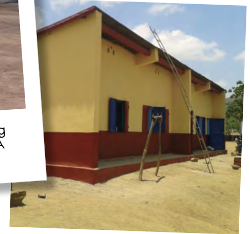
Rehabilitation works at CSB2 Mandiso: Housing for patients' families, latrines, and an incinerator.
